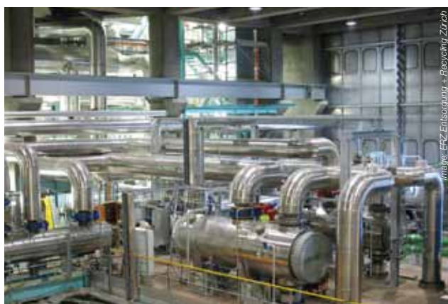
Feeding hot water into the district heating networks: heat condensers in the new Aubrugg wood-fired cogeneration plant.
